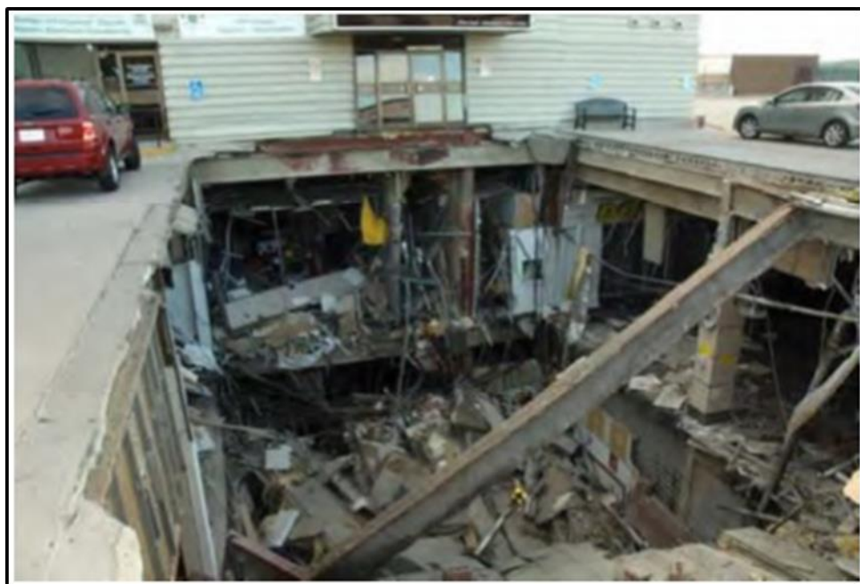
Figure 2.1. Algo Mall Collapse. [Adopted from (McDonald 2013).]
