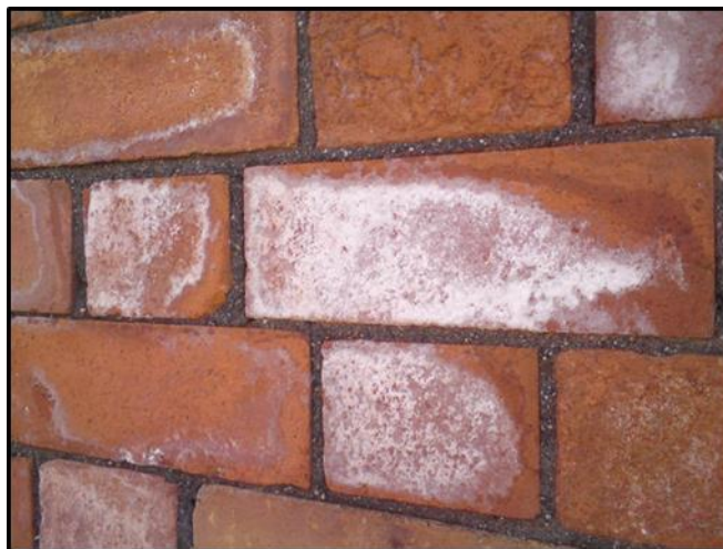
Figure 2.2. Efflorescence effect on red brick.
